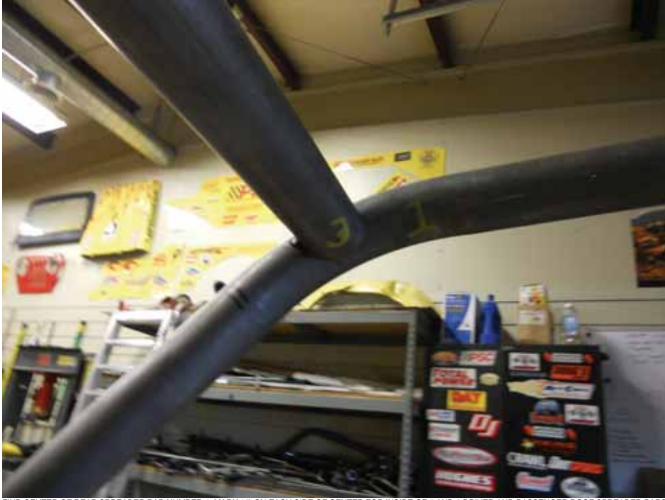
17. FIND CENTER OF REAR SPREADER BAR NUMBER 4. MARK 1/2 ON EACH SIDE OF CENTER FOR INSIDE OF 5 AND 6 DRIVER AND PASSENGER ROOF SPREADER BARS. USE ANGLE IRON OR EQUIVALENT TO FLUSH MOUNT 5 AND 6 TO TOP OF CAGE AND THEN TACK WELD.
